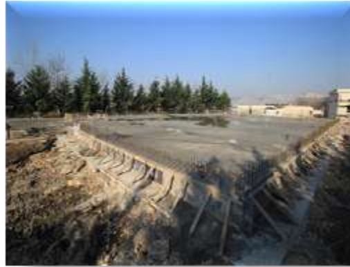
FIRST FACILITY PRODUCING ELECTRICAL ENERGY IN TURKEY Kocaeli Municipality İzmit Water Works Başiskele (Kullar) and Gebze Treatment and Disposal Plant and Energy Recovery Plant
